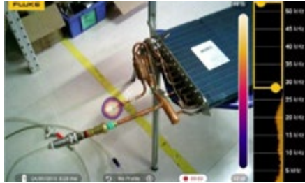
冷媒泄漏检测
